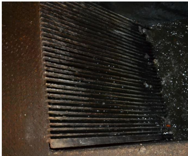
Pic. 1. Manual cleaning grille
